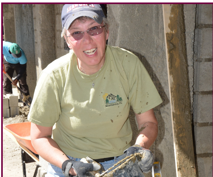
Memory Mission volunteer, Peg Foster, taking her job of building the school wall very seriously!
